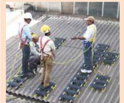
ROOF TOP LADDER
