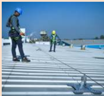
ROOF TOP LIFE LINE
